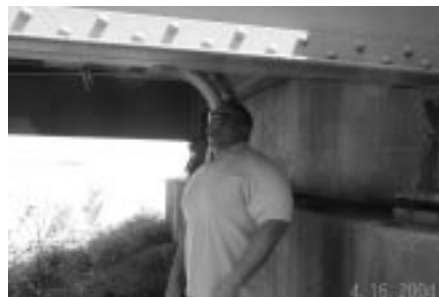
TTAP graduate student Denczil Rolle examines a steel truss bridge as part of a technical assistance project for the City of Dandridge.
