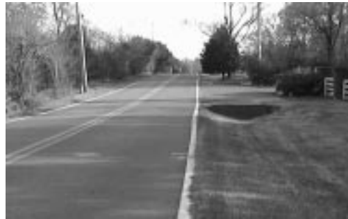
A potential roadside hazard at a new driveway
