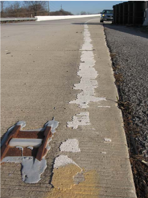
The freeway off-ramp edgeline pictured above is clearly showing the effects of years of damage caused by traffic, weather, and plowing.
