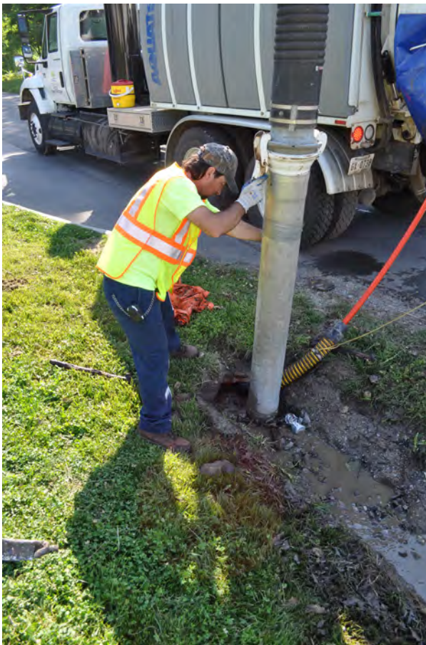
Albert Long uses the vacuum pump to suck up any debris flushed from the drainage pipe.
