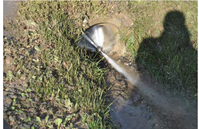
The water jet uses extremely high pressure water to flush out the drainage pipe.
