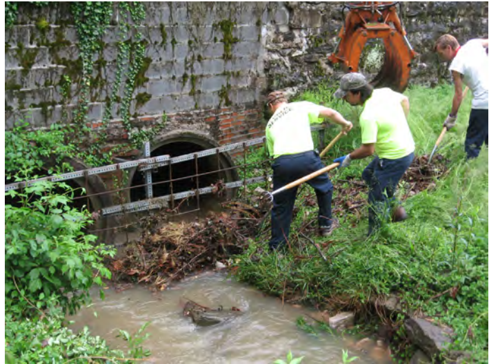
(from left) Danny Hickey, Albert Long, and Tim Tilley work to remove debris from a drainage grate.
