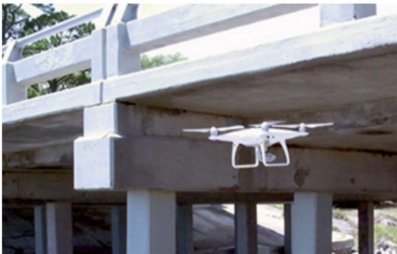
Using Unmanned Aerial Systems for bridge inspections is one of the safety benefits of the UAS initiative from EDC-5. (Source: FHWA)
